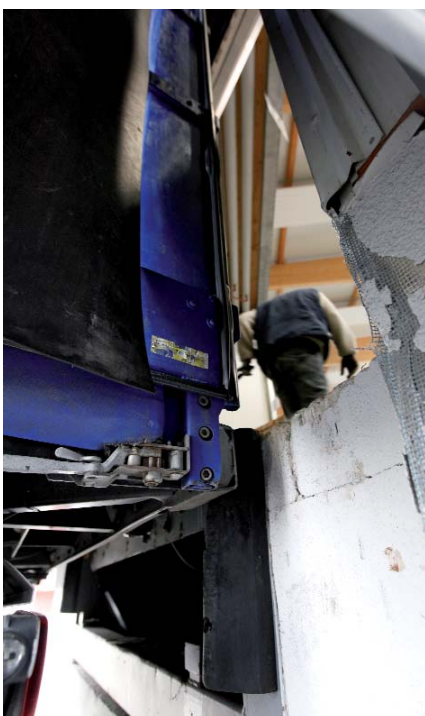
▶ HARD CONTACT LEAVES ITS MARK ON THE TRAILER AS WELL AS THE LOADING DOCK.
